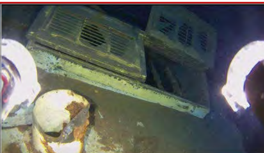
An entrance into the SS Tahoe itself – watch you don't get the tether stuck, though
